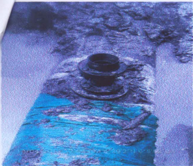
Figure 1: Cut-off Nipple on the pipeline.
